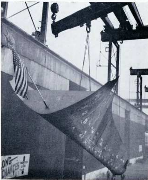
The bow of the S. S. Kernstown being erected. She was Central Yard's first 1944 ship.
