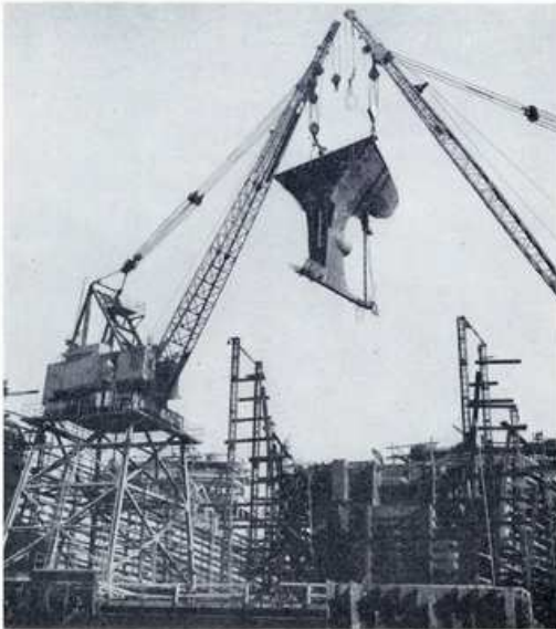
Two fifty ton cranes at North Yard hoisting stern frame assembly in place.
