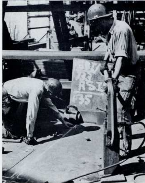
The regulators are pushing the tank top of an interbottom section apart with a hydraulic jack in order to meet their lines.
