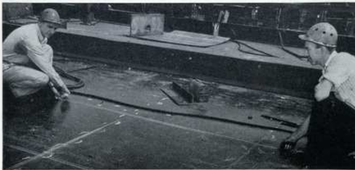
SHIPFITTER FOREMAN E. GATCHEL AND JIM ROONEY laying down set lines for deck house bulkheads.
