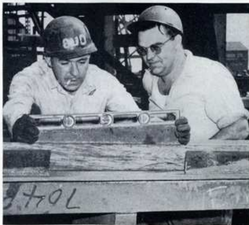
BUD FRANKEL leveling a lube oil service pump foundation as LEADER PHIL LEONARD looks on.
