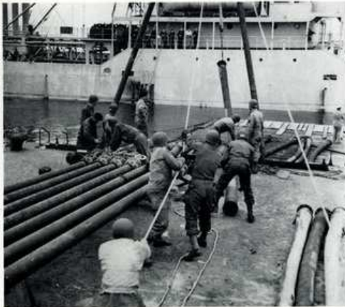
MEMBERS OF AN ENGINEER UNIT make final connections with the ship to shore distribution system for petroleum on the west side of Cherbourg Harbor. The ship, the "Empire Traveller", was the first to discharge its cargo in this manner.
