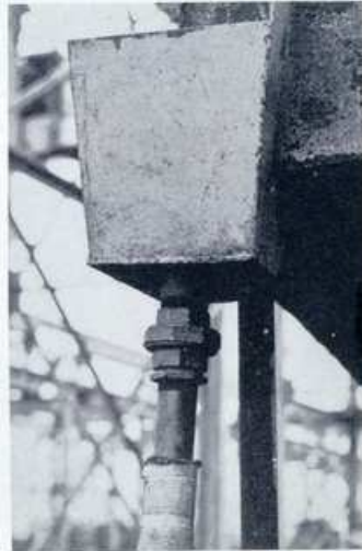
EDWARD HANDLEY, 45-397, won $50 for this Drain Box idea, a specially constructed box which carries the shrinkers water off the decks and increases the factor of safety by carrying the water to the ground before ice is formed on the staging. It also prevents interference with welders on decks, shell butts, and in tanks.
