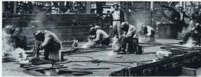
SIX WELDERS working on one butt. A very unusual sight in the Yard.
