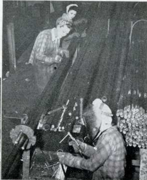
TUBE ELEMENTS being assembled preparatory to automatic fin welding by Kay Arcus and Caroline Petrillo. Tack welding is being done by Phylis Martin.
