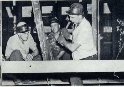
REGULATORS ADJUSTING SIDE SHELL FRAMES to proper position above tank top. L. Wilson, Ass't Foreman II; W. Marnie, Regulator 1st class and T. Fine, Regulator 1st class.
