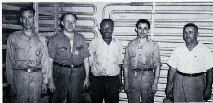
MEAT ROOM with the latest type refrigeration installed on a Sun Ship tanker built in South Yard. Part of the installation crew, left to right: V. Wilson, Leader; C. Miller, A. Powell, M. Rosenthal and L. R. Talley.
