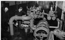
IN FOREGROUND is the emergency fire pump, three stage 1000 gallons a minute, which will build up to 120 pounds pressure. In background are four service pumps which keep the fire lines full of water and supply river water to various sections of the plant. L. to R. John Ogden, Fire Marshal and Robert L. Brown, machinist pumpmen.
