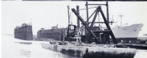
WATER FRONTAGE BEING DREDGED , dredger draws the elements in West Basin east of the Drydocks. Here on case No. 1, the dredger pulled out coal embedded beneath the pier so that this dredger can dig out the coast. No. 2 shows how booms the dredger and No. 3 pictures actual work of excavating the mud and depositing it in a barge.
