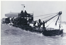
1920 REPAIRING SERVICE. Floating pier being towed on the water. Section will extend from the ship alongside and across the beach. Here the work is being carried out in a temporary pier.
