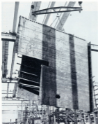
THIS FABRICATED SECTION which was assembled and put together by the ship workers is to be placed on one of the floats, for ship building here of these vessels.
