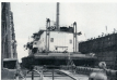
FRANKLIN — Hull and general design, partially drydocking and under-deck repairs and painting.
