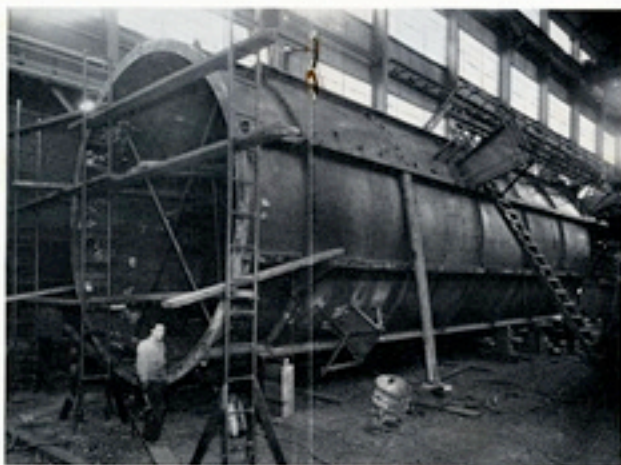
ONE 18' 5 1/2" O.D. x 64' 3" ISO FLOW FURNACE in Boiler Shop.
