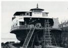
PERSEPOLIS WARSHIP — Drydocking, installation of new shafting, repairs to rollers and other under-deck work.
