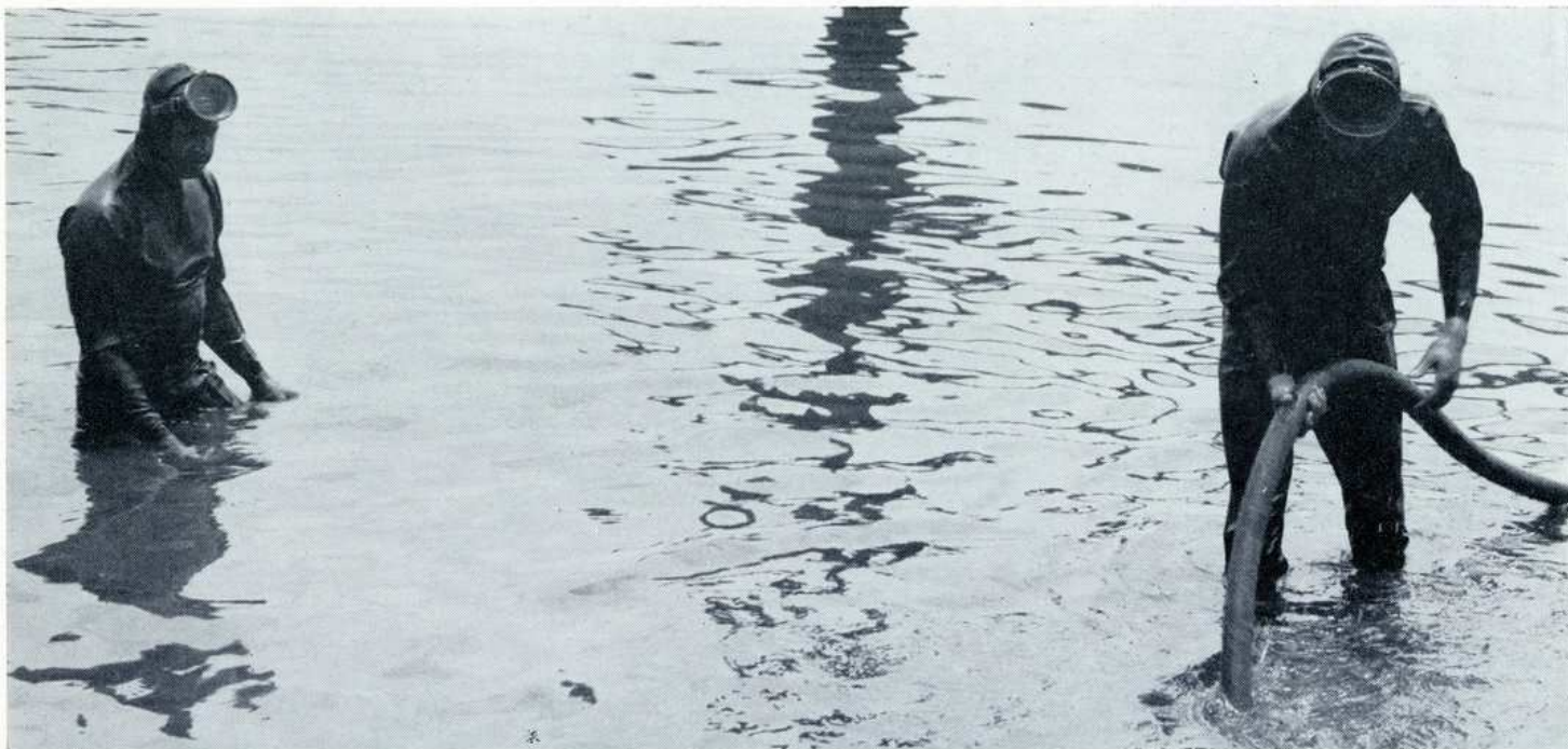
CONSTRUCTION OF RIVER END OF #8 SHIPWAY has necessitated use of skin divers. Above, Lawrence Mayer (left) and Richard Kushto are changing map of riverbottom with a high-pressure air hose. It is difficult to show in a picture of this sort of thing just what is going on, but rest assured they know what they're doing. . . . (see below)
