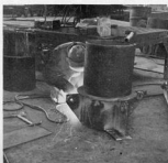
Welder puts finishing touches on one of the four spud caps. After the pipe spud is driven through the spud well of the pier section into the bottom sand, the cap is fitted into the top and the lifting gear attached so that the unit pulls itself up out of the water.
