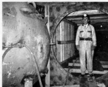
78" diameter tunnel-type mine door for 778½ P.S.L. working press being installed in a stop at the Ogdensburg Mine.
