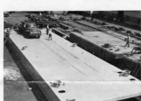
A truck loaded with a two-ton weight was used to test local deflections on the deck of the completed 89' unit. Half of the second 89' unit is in the background.
