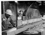
After being moved from plates, the stiffener "blanks" was taken to the Boiler Shop where they were form pressed. Special end cuts were then required before their installation into the various subassemblies.
