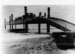
Two small "Doc Ammi" pier sections in the raised position in the surf at Virginia Beach. Winches and hoisting gear are still in place on the inshore unit. The ramp in foreground was not part of contract.
